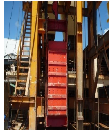
Auxiliary shaft hoist cage
