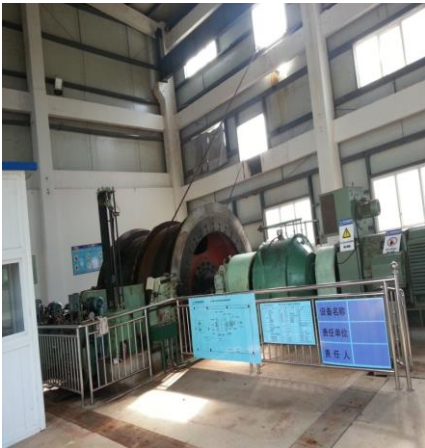
Main shaft Hoist room
