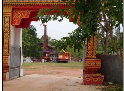
Drilling in the village square at Natan Project, Laos – looking through temple gates
